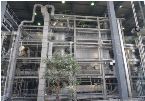
Nake Waste Treatment Plant
